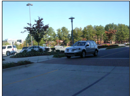
A raised crosswalk connecting a parking lot to a storefront, but lacking paint markings that would increase visibility
