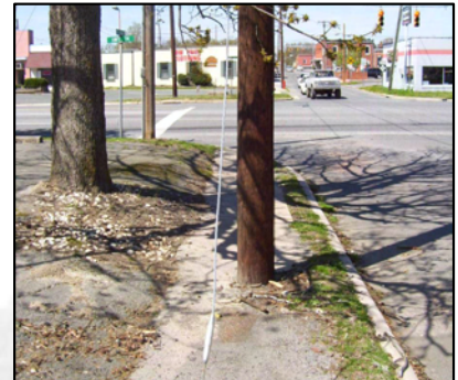
Existing sidewalks have obstacles and maintenance issues.
